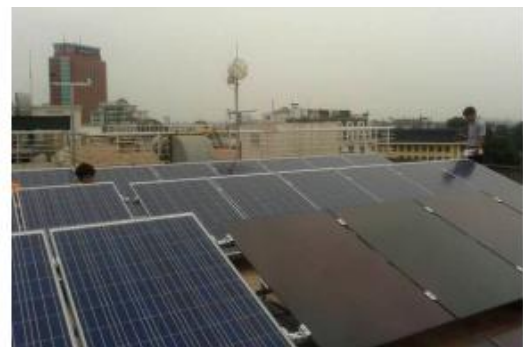
Figure 13. GDE building solar PV system [25]
